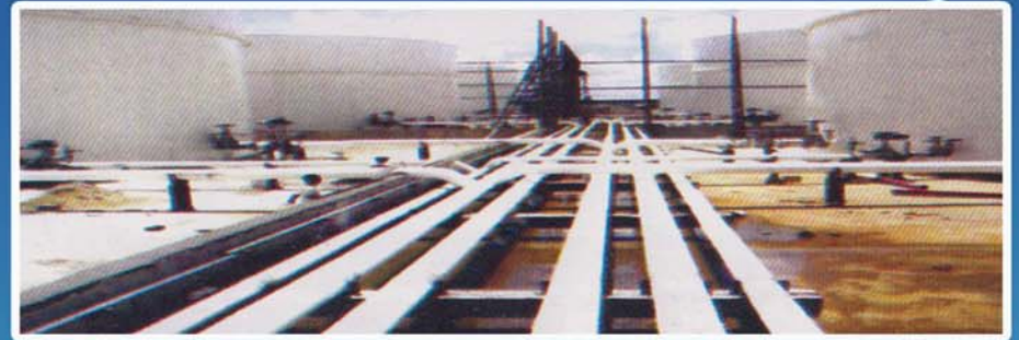
4 ML FUEL STORAGE TANKS AND PROCESS PIPE LINE (ASIA WORLD CO.)THILAWA
