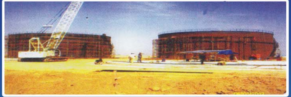
FUEL STORAGE TANKS ( 2 MILLION ) MYAT MYITTA MON CO.THILAWA
